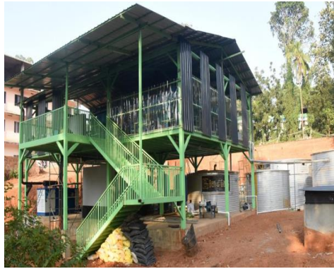
1 MLD STP at Kozhikode medical College
