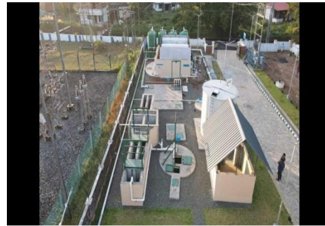
1 MLD CSTP at Padanappalam, Kannur
