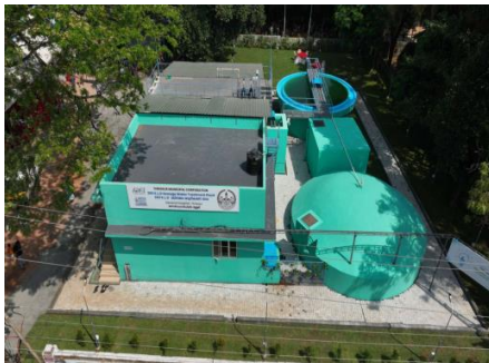
360 KLD STP at General Hospital, Thrissur
