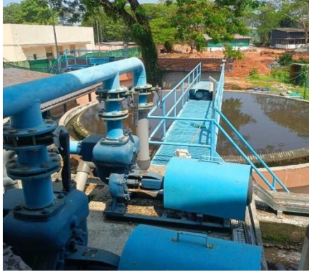
500 KLD STP at Kozhikode medical College
